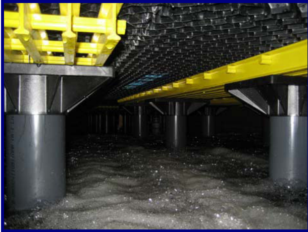
Figure 6 Diffuser under clear water testing during startup
