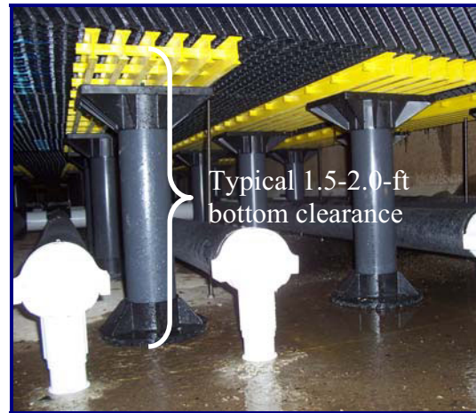
Figure 6 Bottom clearance of media towers showing diffuser ends
