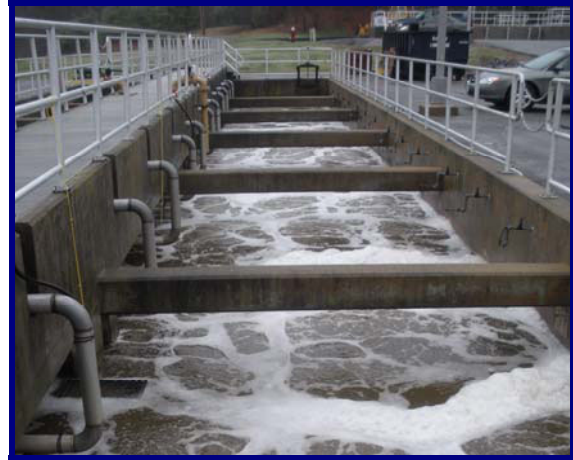
Figure 7 Submerged media towers under aeration
